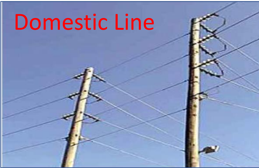
33 to 400 KVA Hightension Line
